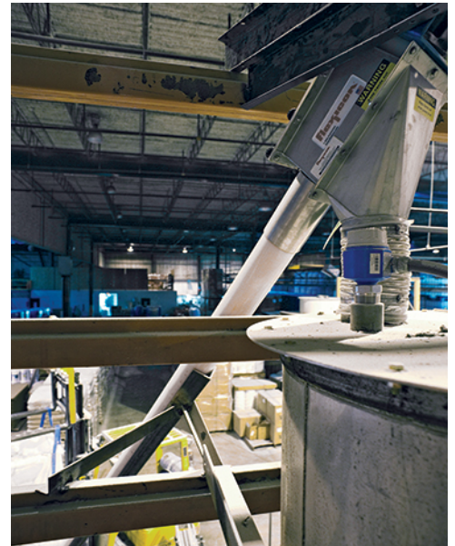
Material discharges from the conveyor tube through a transition adapter into the surge hopper.
