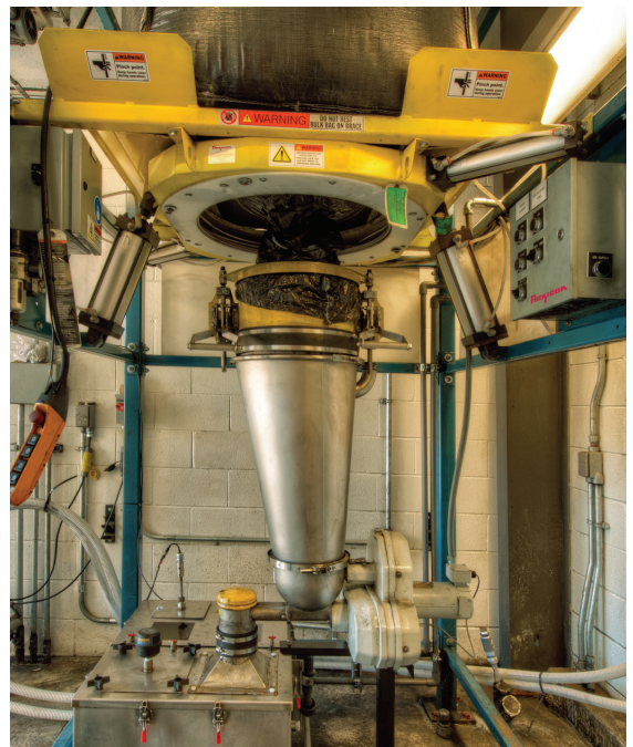
Loaded and flowing: powdered activated carbon flows from the bulk bag to the volumetric feeder and into Consolidated Mutual Water's treatment system.
