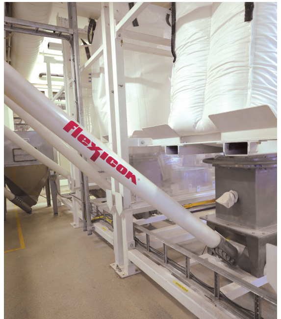
Where gravity feeding of materials is possible, the plant transfers bulk materials using bulk bag dischargers, flexible screw conveyors, rigid augers and pneumatic conveyors.
