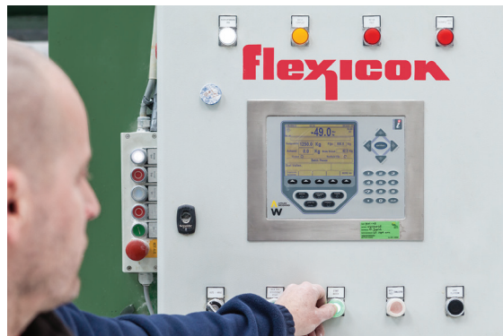
At the control panel, the operator programs the weight to be filled, and initiates the filling cycle. Load cells supporting the filler frame transmit weight gain information to the PLC, which closes a pneumatic slide gate valve when the bag achieves its target weight.
