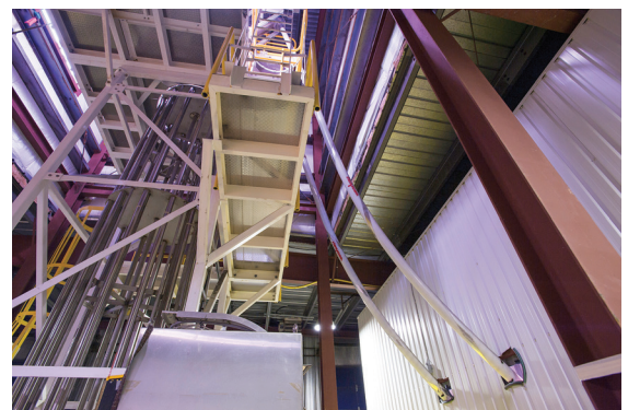
The flexible screw conveyors pass through the wall and then up 36 ft (11 m) to the carousel that fills the Buttbuster tubes.
