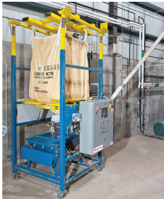
The system controller receives loss-of-weight information from load cells supporting the discharger frame, and stops the flexible screw conveyor once the target batch weight has been lost.
