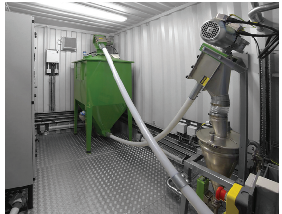
The curved 3.5 m long flexible screw conveyor moves powder from the green surge hopper to the intake of the ejector (right).
