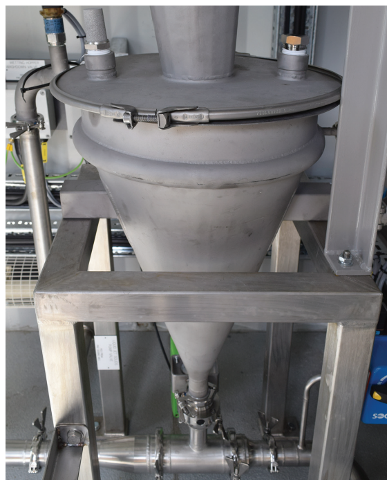
The ejector mixes and doses the slurry of powdered activated carbon into the municipal water stream.
