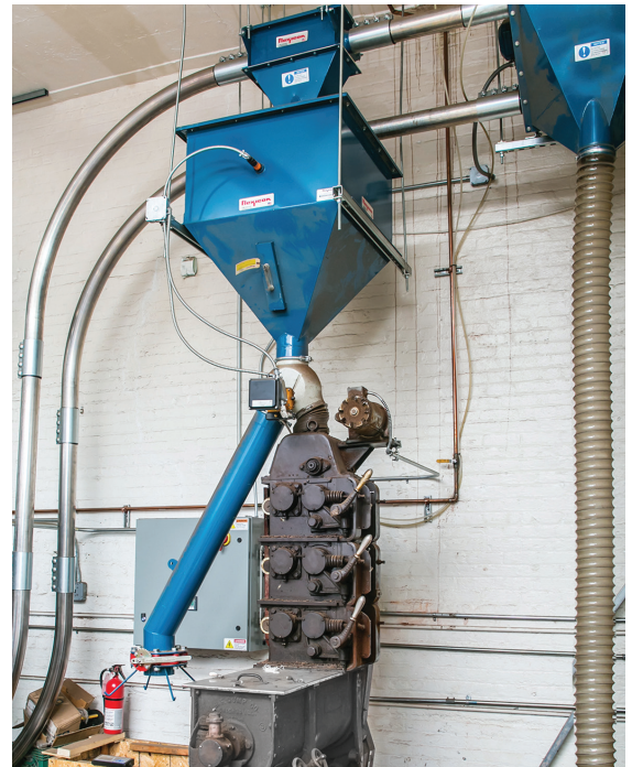
A surge hopper receives roasted beans from the blender via the second TCC line. At left, beans gravity feed through the blue downspout for manual bag filling of whole bean blends. At right, the roasted beans flow to a grinder in preparation for degassing.
