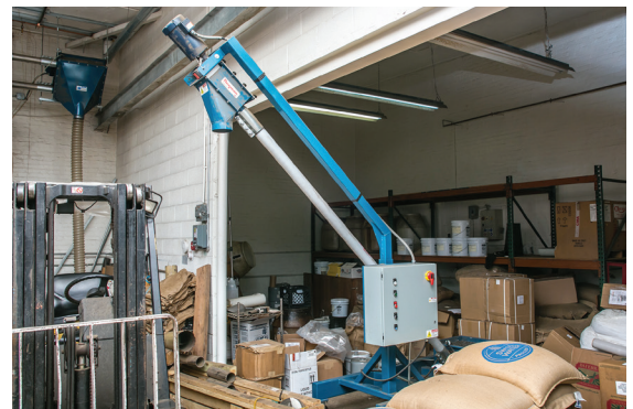
Able to be located off-line until needed beneath the grinder, a portable flexible screw conveyor is used to transfer ground coffee into bulk bags.
