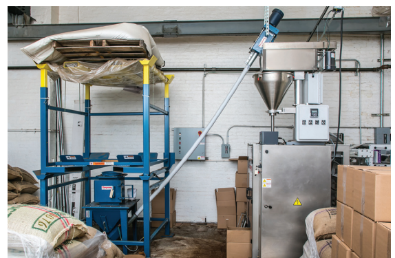
After degassing overnight, ground coffee is discharged from a bulk bag on the split-frame bulk bag discharger while the flexible screw conveyor transfers the coffee to the packaging machine.
