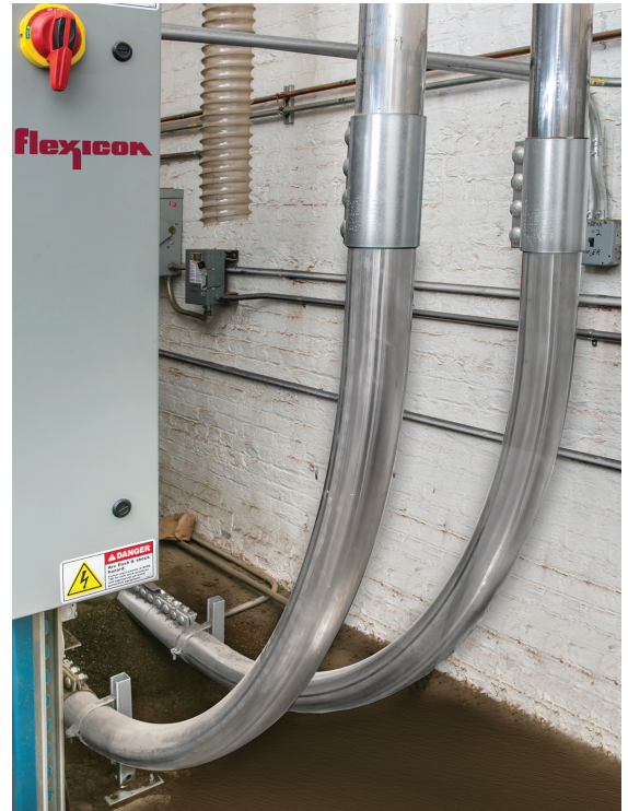
The transfer of coffee through both TCC circuits is controlled by a PLC.
