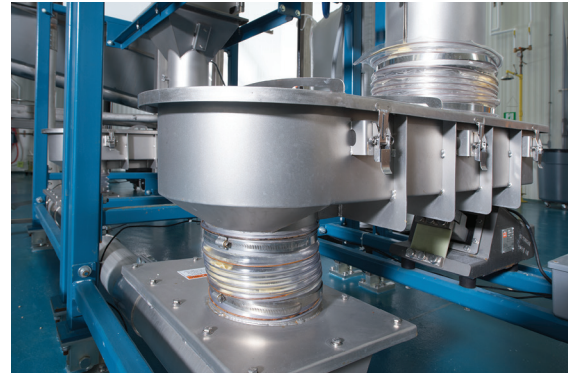
Major granola ingredients enter the TCC line from the bulk bag dischargers through vibratory feeders.
