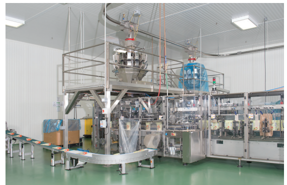
The second TCC circuit supplies surge hoppers of two granola packaging machines through inline tubular discharge valves.
