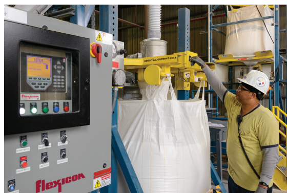
At the bulk bag filler, an inflatable collar seals the bag spout to prevent the escape of dust, after which the PLC inflates the bag to remove creases prior to filling.
