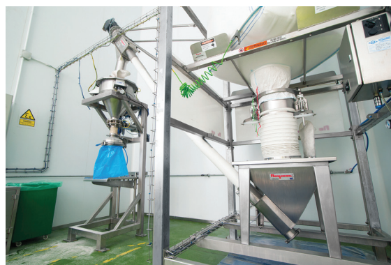
A flexible screw conveyor moves granular sugar from the bulk bag discharger to a gain-in-weight hopper.
