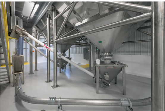
From each transfer bin, a flexible screw conveyor transports peanuts to a pneumatic conveyor line terminating at the final grinding phase of the process.
