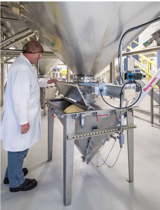
From each transfer bin, a flexible screw conveyor transports peanuts to a pneumatic conveyor line terminating at the final grinding phase of the process.
