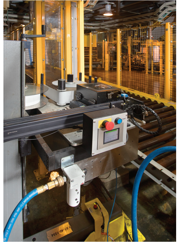
The pallet dispensing and bulk bag filling systems are equipped with automated controls, safety systems and guards.
