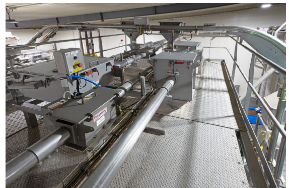
In-line valves allow three TCC systems to intersect and route almonds from a single source to multiple destinations, depending on needs. The valves open to discharge almonds into a predetermined destination (below right) or remain closed to allow transport toward other processing functions (below left).
