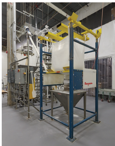
Blended material flows from a bulk bag into the floor hopper of a flexible screw conveyor, which discharges into a vibratory separator discharging into a packaging machine.
