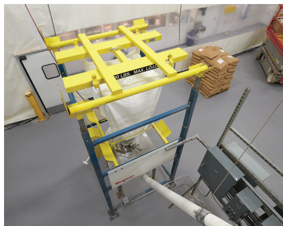
A forklift places the bag and lifting frame onto the Bulk-Out® BFF bulk bag discharger frame.
