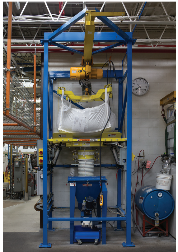
In delivering "flour" to the process, a lifting frame, cantilevered I-beam, trolley and hoist place the bag in the discharger frame. Flow-Flexer® bag activators (top corners, lower half of frame) promote flow as the flour tends to bridge.
