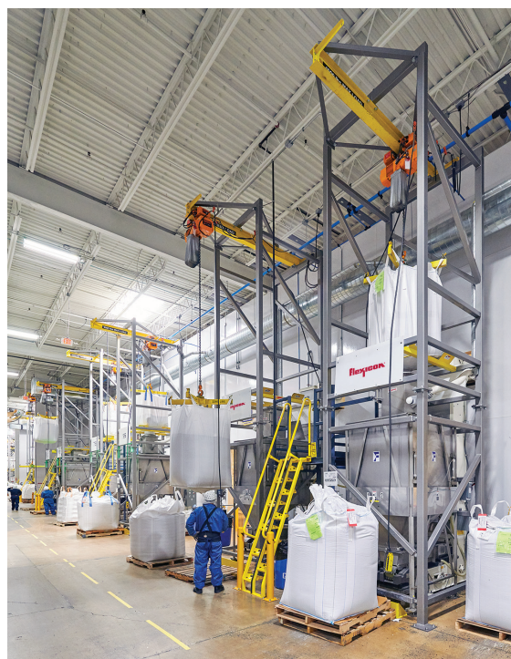
Bucket conveyors move material from 12 bulk bag dischargers through the wall of a packaging room.
