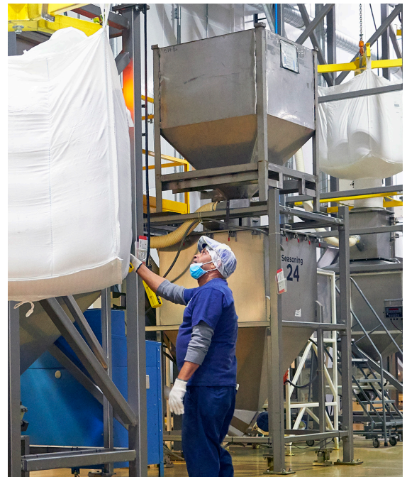
Flexible screw conveyors transfer flour from bulk bag dischargers, and rice mix spices from a rigid tote discharger, through small openings in a wall separating the warehouse from a packaging room.
