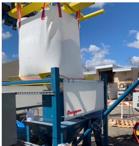
A fork truck holds the bulk bag over the half frame discharger while the flexible screw conveyor moves sodium bicarbonate to the mixing tank.
