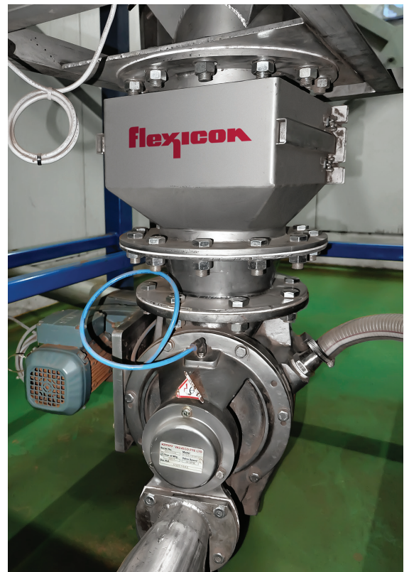
A rotary valve meters presscake into a pneumatic conveying line that discharges into a storage silo.
