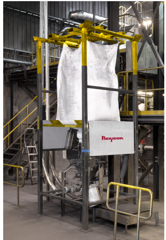
A rotary valve beneath each hopper feeds graphite to a tubular cable conveyor, which gently moves it dust-free to a jet mill for fine grinding.
