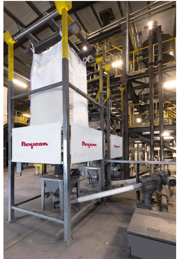
From hoppers beneath each bulk bag discharger, flexible screw conveyors introduce raw graphite into a tubular cable conveyor, which gently moves it to a jet mill on the mezzanine.
