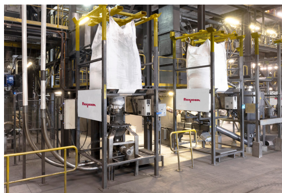
Pairs of forklift loaded bulk bag dischargers feed raw graphite into tubular cable and flexible screw conveyors which transport it to silos and the milling process.
