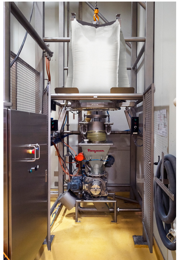
Bulk bag dischargers meter major ingredients by weight into a pneumatic line. Bags are inserted and removed using a cantilevered I-beam, hoist and trolley.
