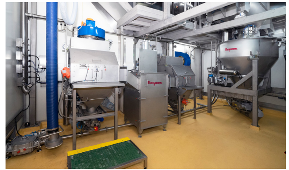
Twin bag tip stations for adding low volume ingredients flank a bag compactor which compresses empty bags for dust-free disposal. The large buffer hopper (right) receives blended batches that are transferred pneumatically to the downstream process.
