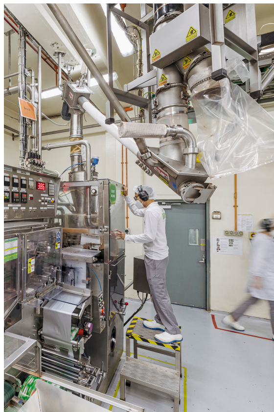
Contaminant-free powder gravity feeds from the raised metal detector (top-right) and is transported by the flexible screw conveyor to the sachet filler.
