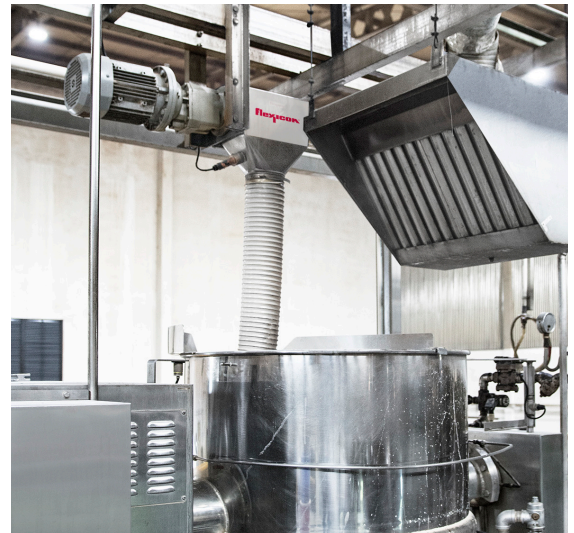
Another filter receiver intakes sugar and discharges it into a receiving hopper which supplies the packaging line. Tereos Sucre chose pneumatic conveying to eliminate the risk of contamination.
