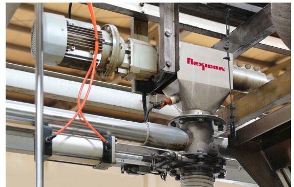
Sugar gravity feeds from the flexible screw conveyor through downsputting into a juice cooker. The motor is positioned beyond the conveyor discharge, preventing material from contacting bearings or seals.
