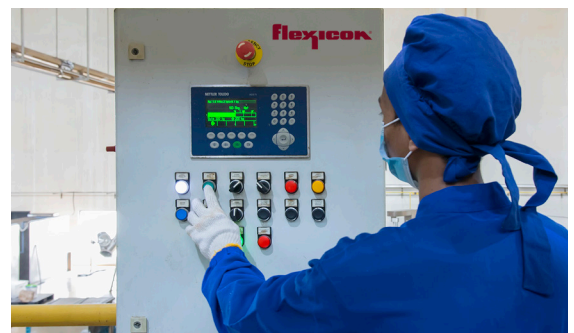
Under PLC control, the system weighs and delivers sugar to the six juice cookers at high rates.
