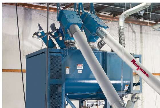
From two bulk bag dischargers, two large diameter flexible screw conveyors transport talc and graphite to the blender while the 80 cu ft (2265 l) surge hopper feeds the blended batch into two smaller flexible screw conveyors supplying two packaging lines.
