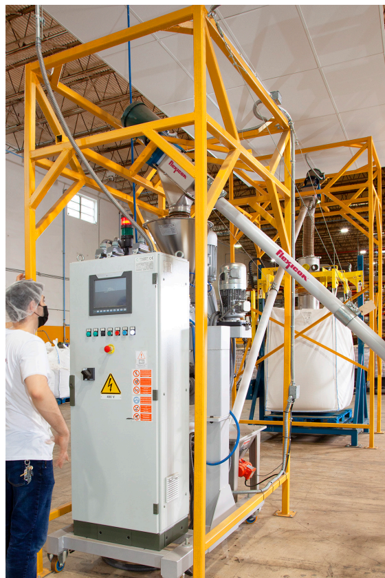
Flexible screw conveyor (top right) transfers beans to the grinder, from which a second flexible screw conveyor moves ground coffee to the bulk bag filler (rear).
