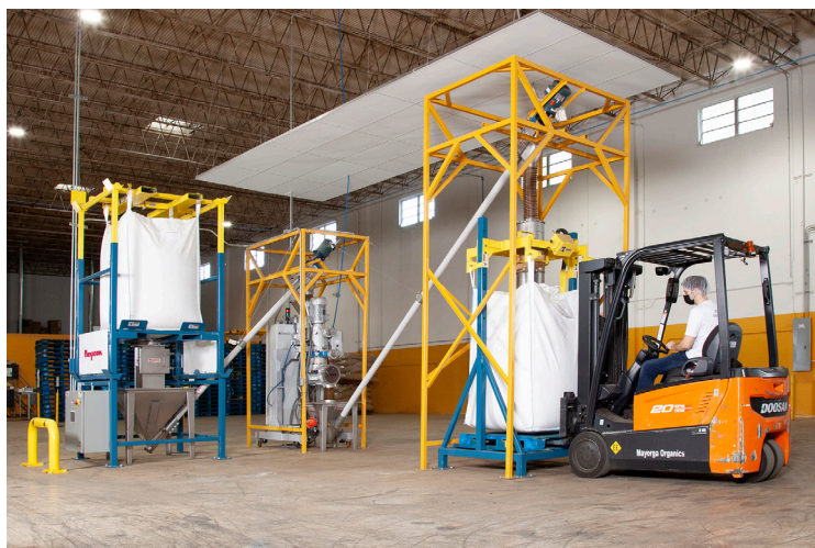
The flexible screw conveyor at left transfers roasted coffee beans from the bulk bag discharger to the grinder, while the conveyor at right moves ground coffee to the bulk bag filler.
