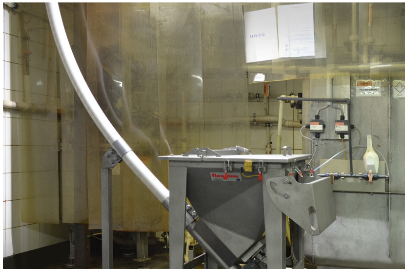
The conveyor exits the hopper at a 45 degree incline and curves to vertical, elevating the material 5.5 m (18 ft) to the dosing system inlet dust-free.
