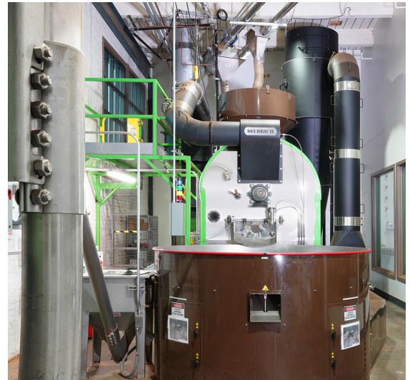
In foreground and top center, the tubular cable conveyor transports and discharges beans into the roaster.
