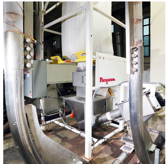
Below the bulk bag discharger, a flexible screw conveyor transfers raw beans into the inlet of the tubular cable conveyor routed to the roaster. Load cells supporting the discharger frame transmit weight loss signals to slow and stop the flexible screw conveyor when the precise batch weight is lost.
