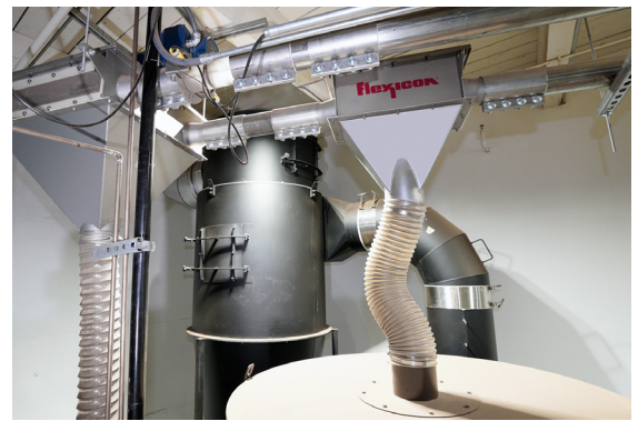
Beans gravity feed from the tubular cable conveyor through a discharge adapter and flexible downspouting into the roaster below.
