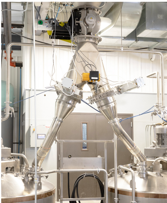
An inline fill/pass valve directs material to one hopper feeding two smaller coolers.
