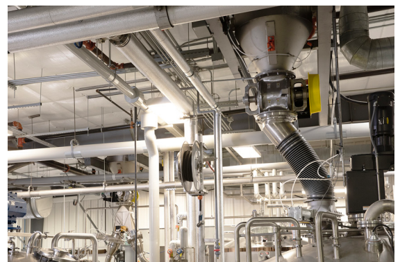
The dilute phase, vacuum pneumatic conveying line transports grain across the facility.
