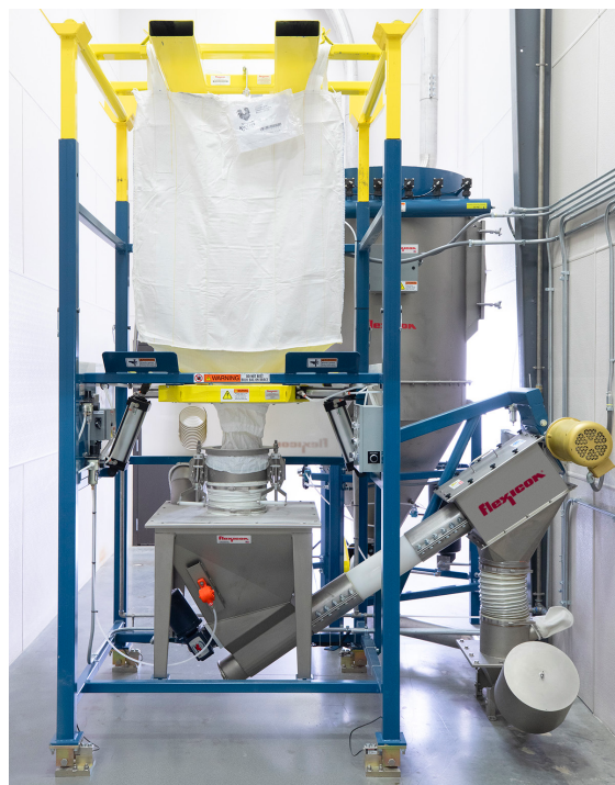
A loss-of-weight bulk bag discharging system with integral flexible screw conveyor feeds grain by batch weight into a Flexicon pneumatic conveying line that, in turn, feeds cookers on the opposite side of the facility.
