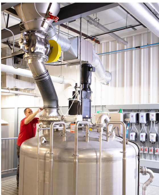
The dilute phase, vacuum pneumatic conveying line transports grain across the facility.
