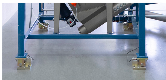
Load cells supporting the discharger transmit loss-of-weight signals to a PLC which stops the flexible screw conveyor when a predetermined weight of grain is lost.
