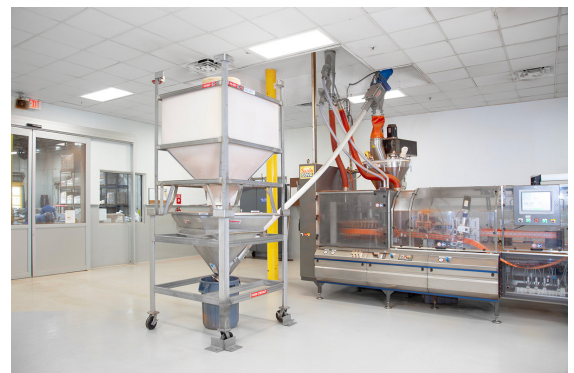
Blended batches are gravity discharged into a polymer surge hopper and flexible screw conveyor that feeds a packaging machine with no separation of blends. The fully enclosed system prevents contamination of the product and plant environment.
