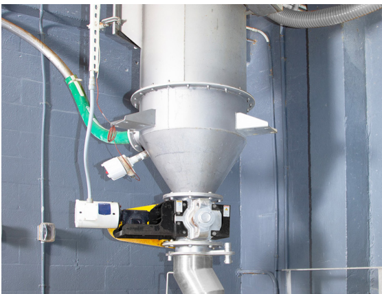
The filter receiver discharges through a rotary airlock valve into the blender below.
