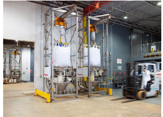
Five identical bulk weighing and batching systems, each comprised of a bulk bag discharger on load cells, move ingredients from bulk bags through a pneumatic conveying line to five blenders.
