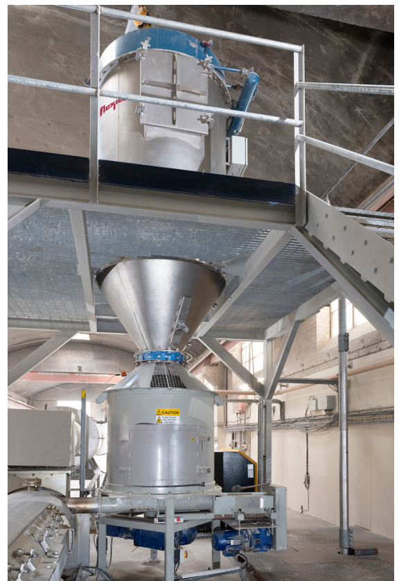
The hopper below the filter receiver receives the wet mica and discharges it to a drying system followed by separation by particle size.
