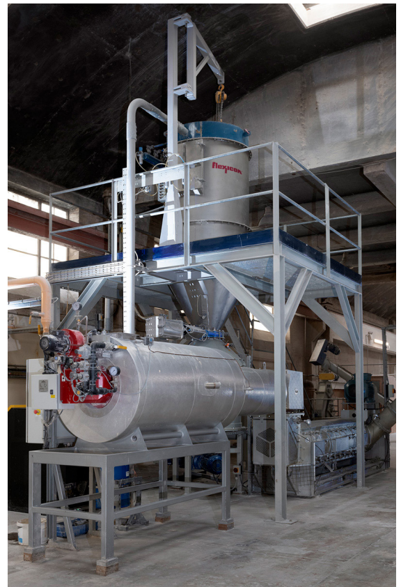
A 30 m (98.4 ft) long conveying line transfers wet, abrasive mica powder from the wet process on the floor below into the filter receiver which separates the material from the conveying air.
