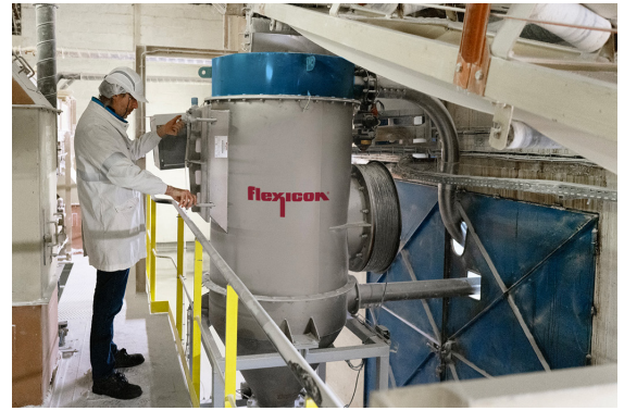
Another filter receiver intakes sugar and discharges it into a receiving hopper which supplies the packaging line. Tereos Sucre chose pneumatic conveying to eliminate the risk of contamination.
