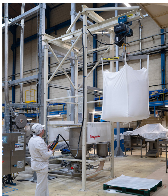
Using a pendant, the operator hoists a bulk bag of extra-fine sugar along the cantilevered I-beam into the discharger frame.
