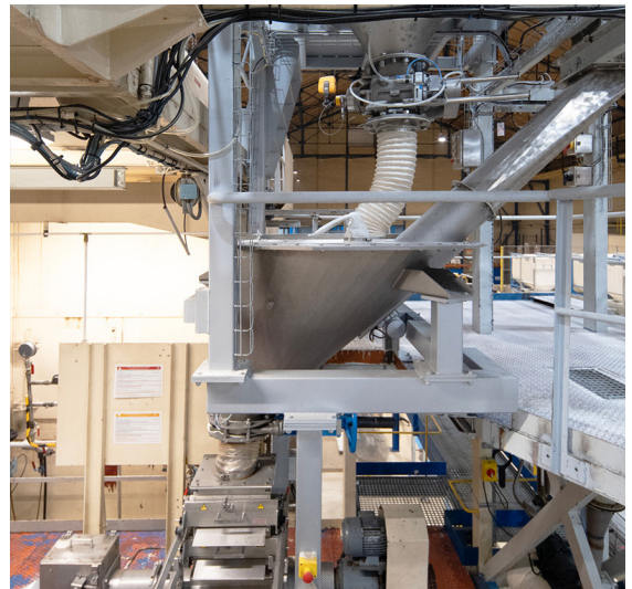
A dual pipe plug diverter directs sugar either 20 m (65 ft) to the wet process for sugar cube production, or 8.5 m (28 ft) to the packaging line.
