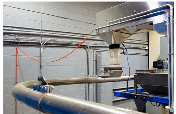
At the rear of the building, beans from the roaster are discharged from a bucket elevator into the Tubular Cable Conveyor.
