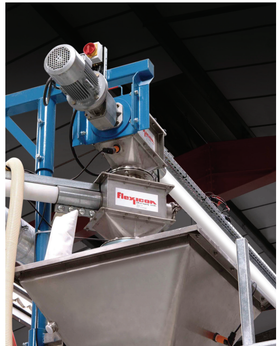
At first of three transfer points, slide valve between flexible screw conveyor and hopper inlet opens/closes to regulate product flow.
