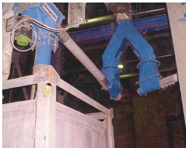
Pulverized fuel ash transfers through bifurcated chute assembly and flexible screw conveyors to two weigh silos for transfer to sluice valve hoppers.
