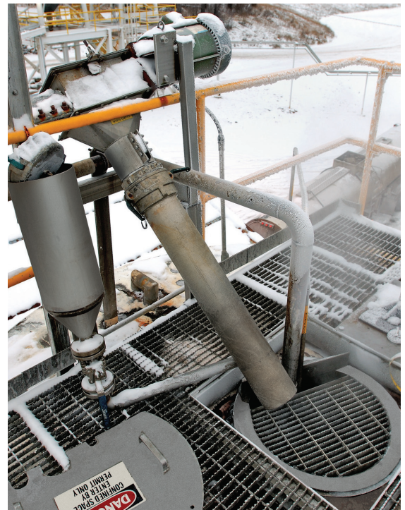
Material passes through the diverter valve and is charged to the first blending tank through a delivery tube.
