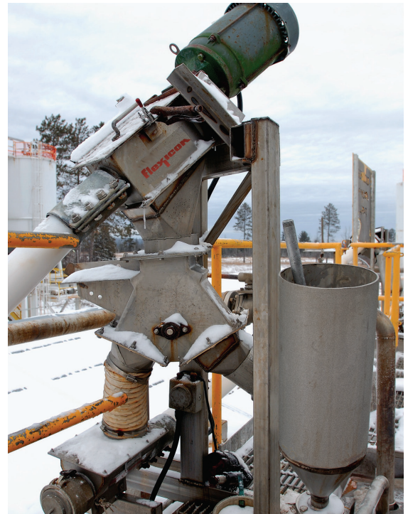
A diverter valve directs material from the second conveyor directly into one blending tank, or into a third conveyor that discharges into another tank.
