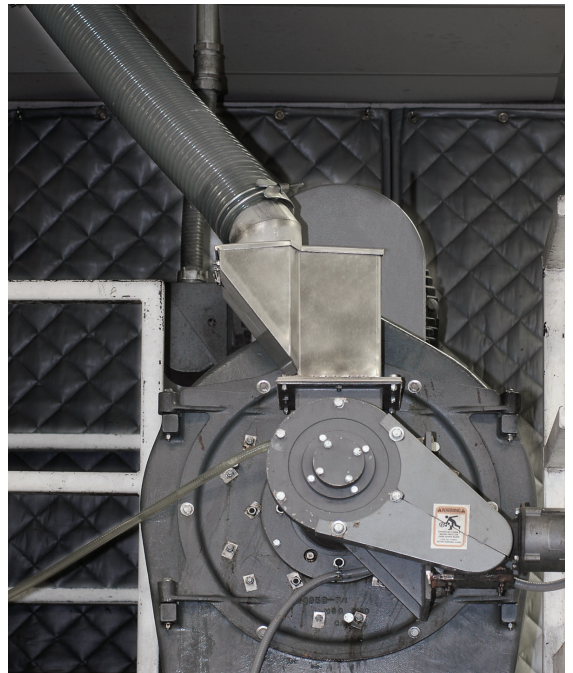
A flexible screw conveyor discharges raw nuts through a transition adapter and downspout into the main process mill.
