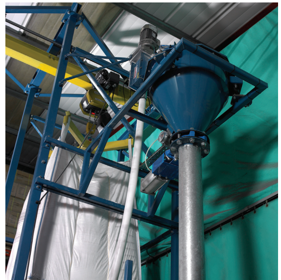
A flexible screw conveyor (the narrow tube in the middle of the photo) transfers product to the weigh hopper, which is mounted on load cells that transmit gain-in-weight information to the control panel.
