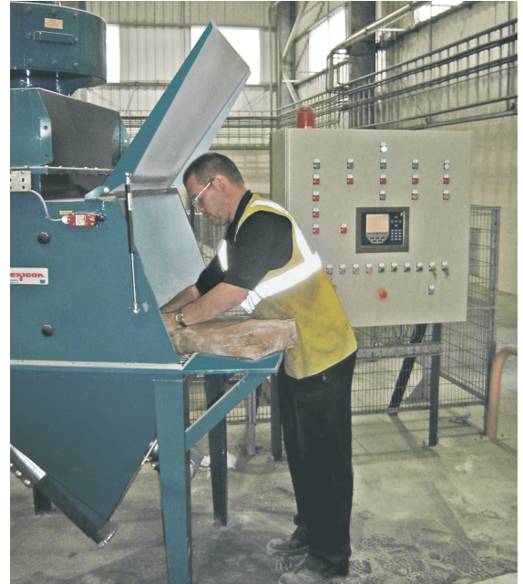
Dust generated by operator splitting and dumping of bags is contained by dust collector of bag dump station.
