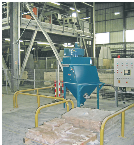
A 30 ft (9 m) long flexible screw conveyor transfers aluminum powder from a bag dump station to a gain-in-weight hopper on the mezzanine.
