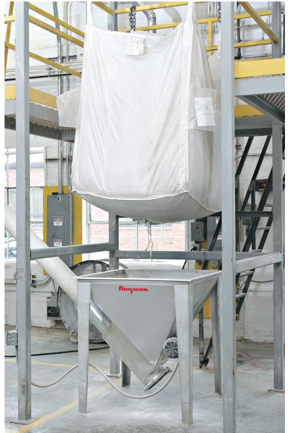
A bulk bag is readied for discharge into the floor hopper. The bottom end of the flexible screw conveyor is below and to the left of the hopper.
