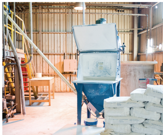
Titanium dioxide travels from the conveyor's discharge spout through a 4 ft (1.2 m) long downspout before entering the blender. A controller achieves batch weight accuracy of \pm 0.02 lb ( \pm 0.01 kg).
