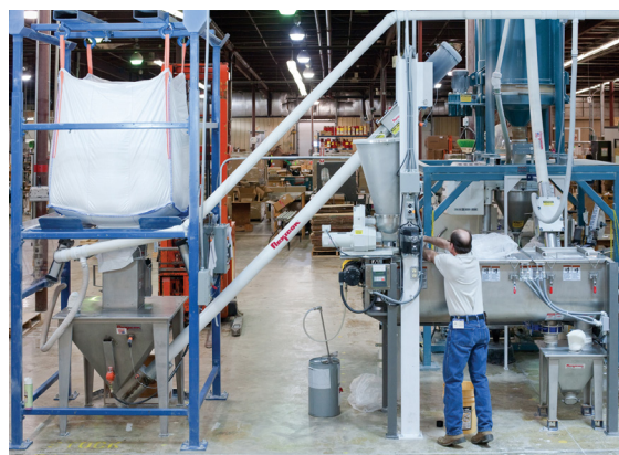
At left, a 10 ft (3 m) long flexible screw conveyor moves talc from hopper beneath the bulk bag to the paddle blender. At right, a 15 ft (4.5 m) long flexible screw conveyor transports the blended batch to the packaging machine. On top, a vacuum line pulls dust into a dust collector.
