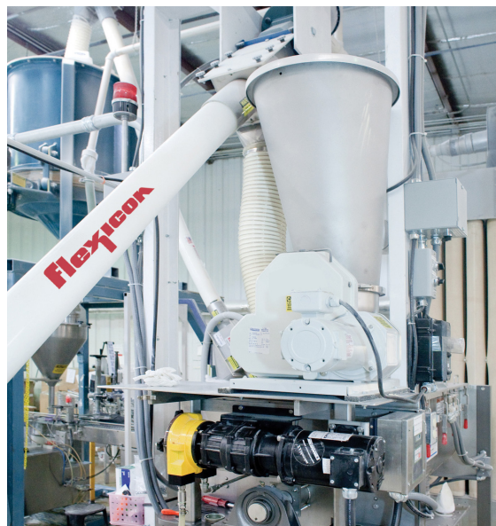
A 10 ft (3 m) long flexible screw conveyor moves talc from hopper beneath the bulk bag to the paddle blender, while a liquid metering pump and bulk solids feeder meter glitter and fragrance oil into the blender.
