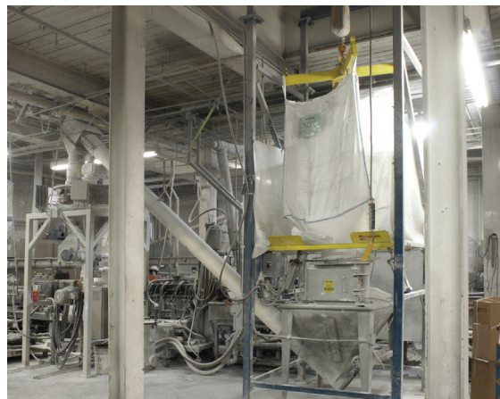
The first bulk bag discharger installed by The Plastics Group has a 6 in (150 mm) diameter flexible screw conveyor that transports material 17 ft (5.2 m) to a feeder hopper on a twin-screw extruder.
