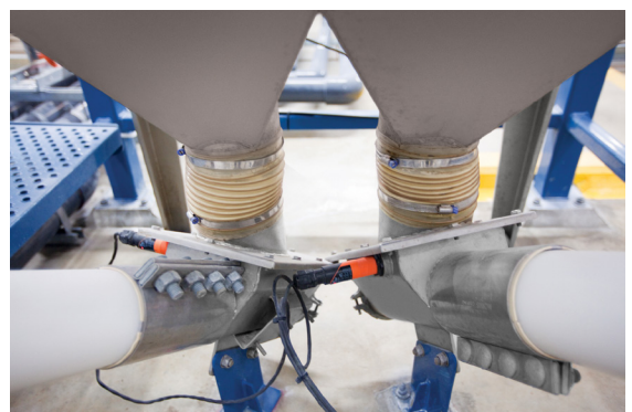
Fluoride powder flows from double outlet hopper through sealed connections to the two flexible screw conveyors that move it to the two storage hoppers.
