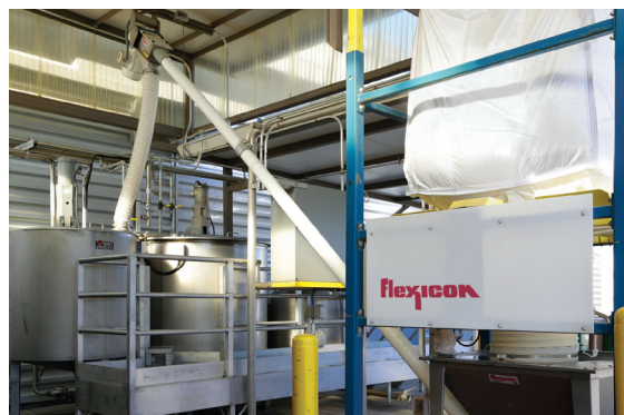
Diatomaceous earth moves from the bulk bag through the hopper, flexible screw conveyor and downspout to a 300 gal (1136 l) tank before filtration of the wine. The completely enclosed system eliminates dust and reduces costs from manual dumping of small bags.
