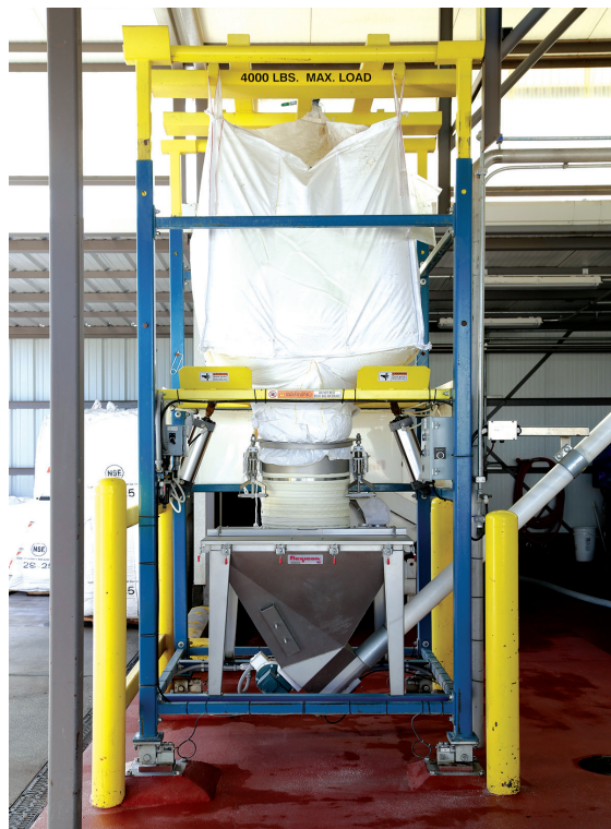
Diatomaceous earth flows from the bulk bag through the dust-tight bag spout interface, hopper and flexible screw conveyor to the holding tank. FLOW-FLEXER® bag activators on opposite bottom sides of the bag promote complete discharge. Load cells allow automated weigh batching.
