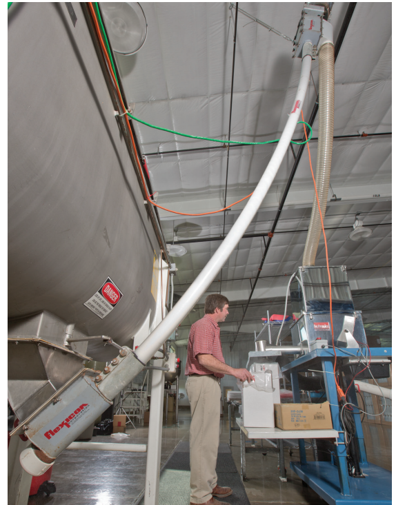
From the blender the mixture enters the intake of the flexible screw conveyor through a transition adapter. Cleanout cap (bottom right) facilitates washdown of the internal spiral.
