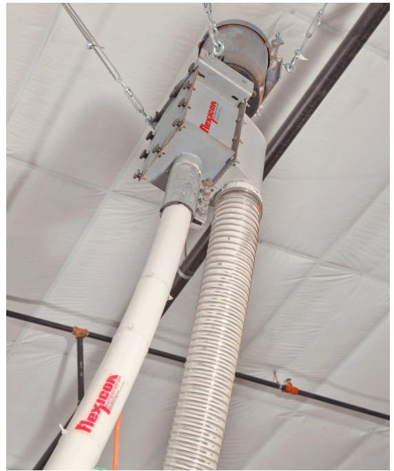
Powder exits the flexible screw conveyor at the drive end and descends through the downspouting to the packaging machine. The transfer is fully enclosed and dust-free.
