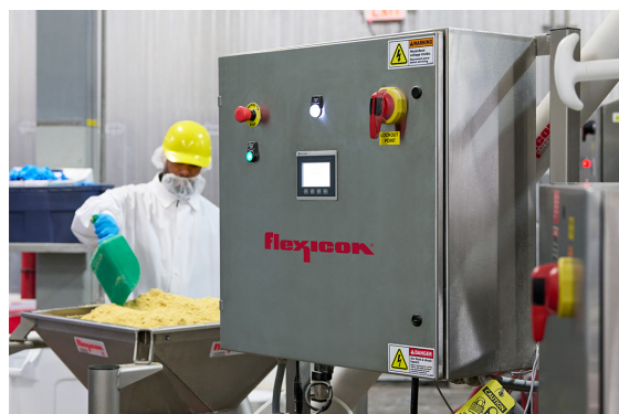
A Flexicon built and programmed NEMA 4X stainless steel control enclosure protects the electrical components during washdowns and in humid environments.
