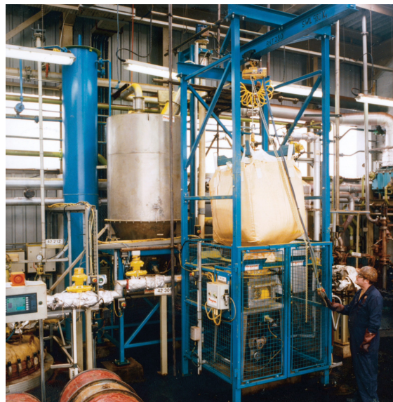
Bulk Bag Discharger working in flammable area, feeding batches of raw material to a reactor vessel.
