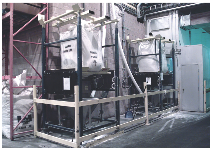
Bulk bag dischargers unload salt (L) and whey (R) from 2200 lb (1000 kg) bags into hoppers equipped with flexible screw conveyors that transport the material to the sanitary room.
