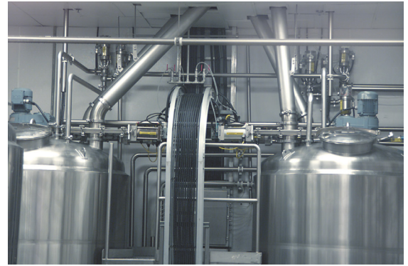
Each diverter valve can direct the salt or whey through drop chutes to either of two raw milk tanks.
