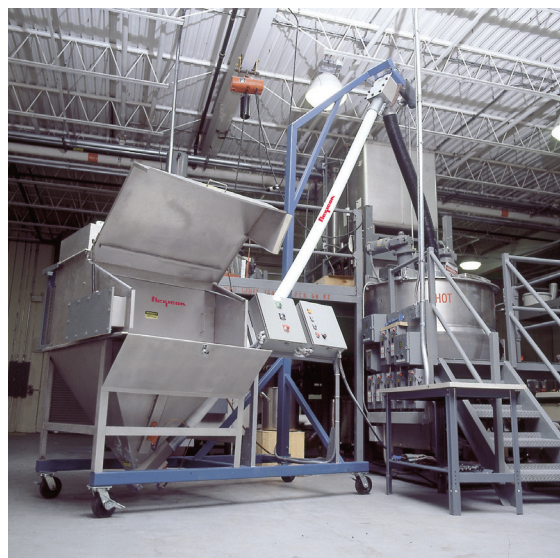
Bag dump station, dust collector and flexible screw conveyor are self-contained on a caster-mounted frame which is wheeled between process vessels requiring 300 lb (135 kg) batches of fumed silica.
