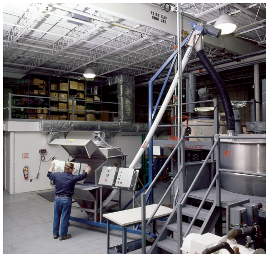
Operator empties bags of fumed silica into bag dumping station dust-free while flexible screw conveyor feeds line material into a process vessel
