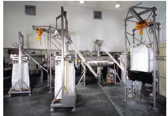
Flexible screw conveyor at right transports dextrose granules from bulk bag discharger at 500 lb (225 kg) capacity blender. Second flexible screw conveyor transports blended powders to the bulk bag filler. Blended powders discharged from the 2500 lb (1125 kg) capacity ribbon blender are transported through a flexible screw conveyor to the bulk bag filler at left. From the bulk bag discharger (shown empty), another flexible screw conveyor will convey powdered flavors to the packaging line.
